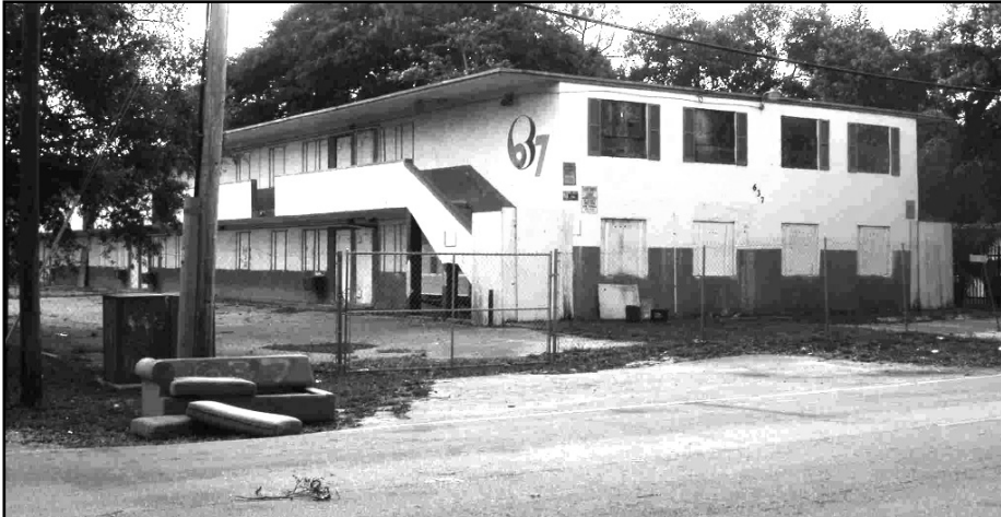
637 SW 15th Avenue has been boarded up since the mid-1990s. The City Commission's action on May 18th paves the way for demolition of the building.
